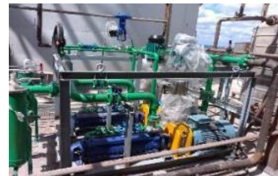
Pump skid feed pump & booster pump
